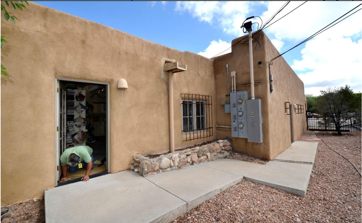
Electric Service & Pole-mounted transformers Southside of the property.
