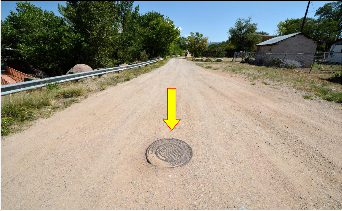
Manhole cover for Santa Fe City Sewer on the Service Road, Northwest of the property.
