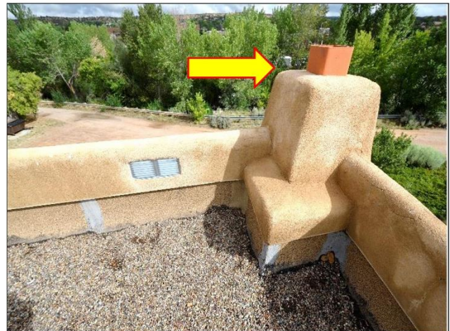
6. Chimneys need spark arrester as per city fire codes.
