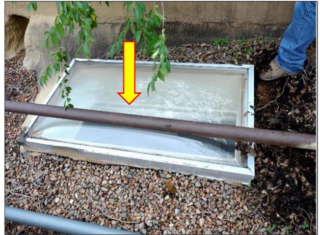
8. Skylight should be removed and/ or gas pipe should be relocated. Curbing is too low and a heavy snow load could cause leaks.
