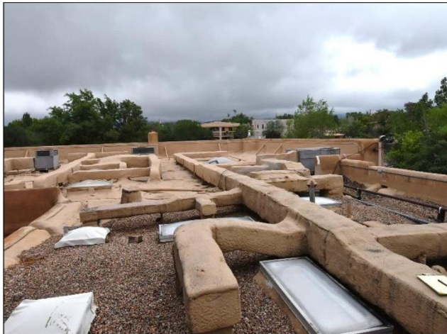
3. Rear Section of foam roof w/ rock on the South Building showing all the ducting needs maintenance to improve on its roofing integrity.
