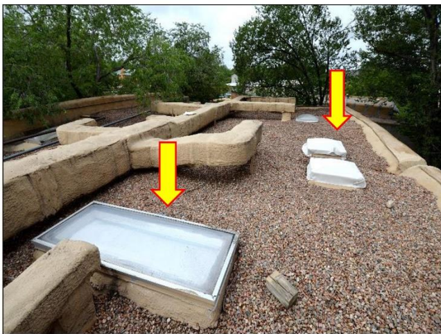
9. All the Skylights on the rear section of the South Building should be raised because the curbs are too low and will leak after a snow fall.
