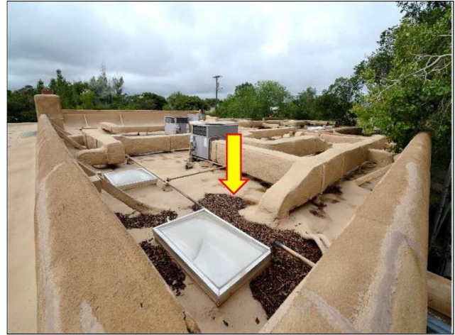
2. South Building Foam & GACO Roof is full of debris and needs a serious clean and a reappointment due to breaches found on the membrane.
