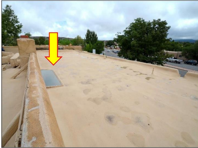
1. South Building Entrance Portal is the Best Foam roof with a longevity of over 20-years. Flat Skylight is questionable.
