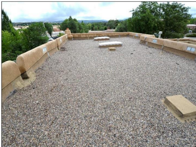
5. North Building Hot/ Tar & Mop roof is in Good Condition with minimal reappointments necessary.
