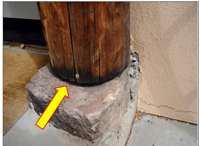
12. Viga post under the North Building Portal need to be grouted for better stability.
