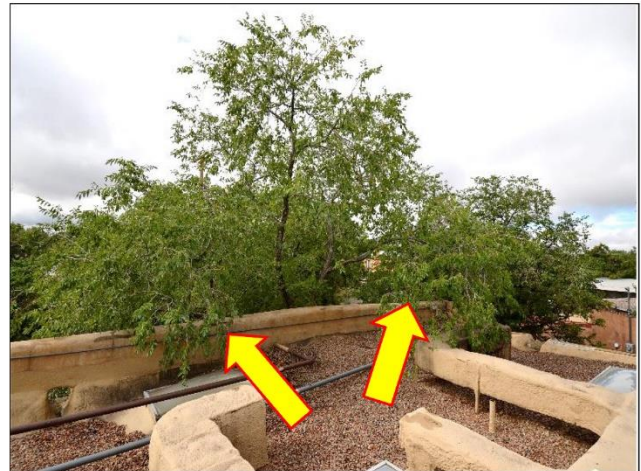
4. Over grown trees needs to be trimmed back to keep their leaves for clogging the drainage Canales on the roof.
