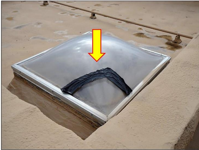
7. Cracked Skylight is tapped and needs to be replaced.
