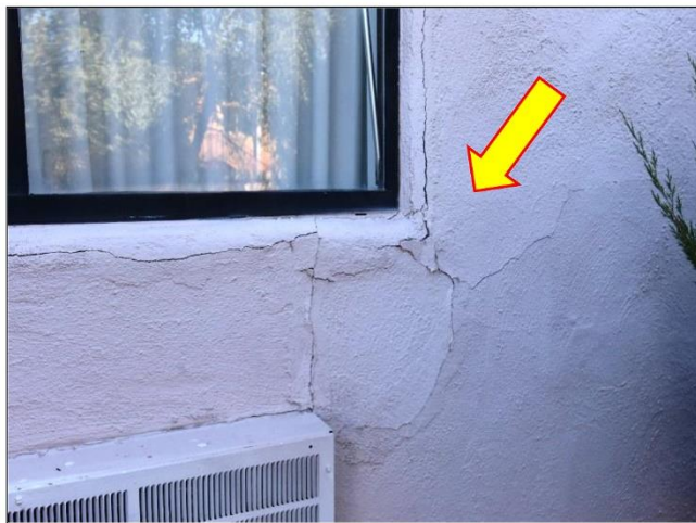
45. Example of some of the worst cracking found around windows, doors and PTAK openings that will need a Stucco repair and Stucco Restoration analysis.
