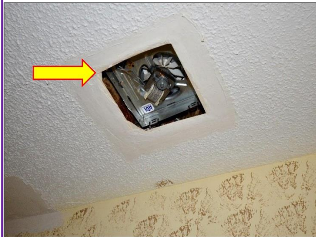
75. Bathroom fan is missing cover and all fans will need to be verified.
