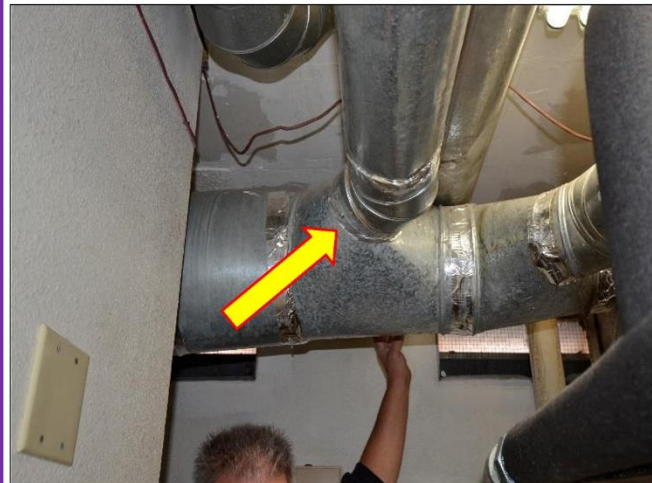
35. The Exhaust flue angle is too high and will not draft properly.
