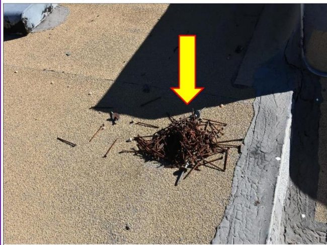
11. Left over nails that are rusted should be removed because they can cause deterioration of the membranes.
