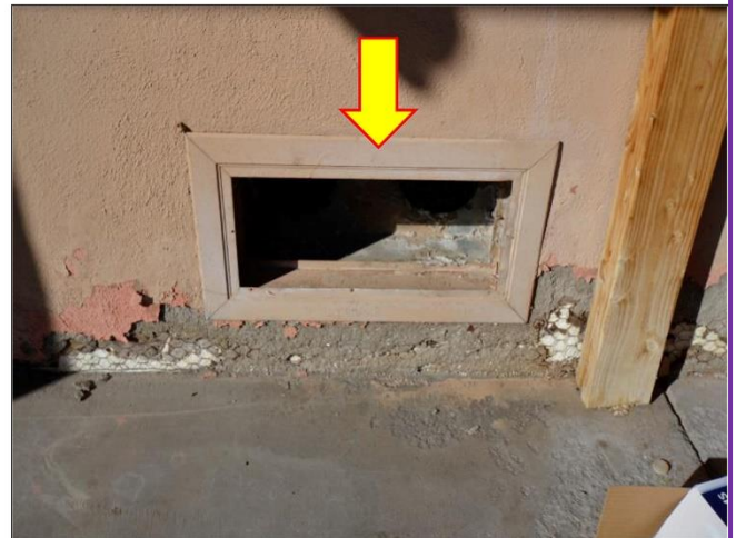
34. Vent opening at the Laundry Room needs a cover grill and the stucco wall below showing exposed lath wire will need to be repaired.
