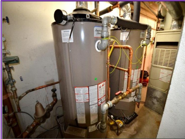
37. Two 100-gallon H 2 O heaters have been properly installed in the 1989 portion of the Building.
