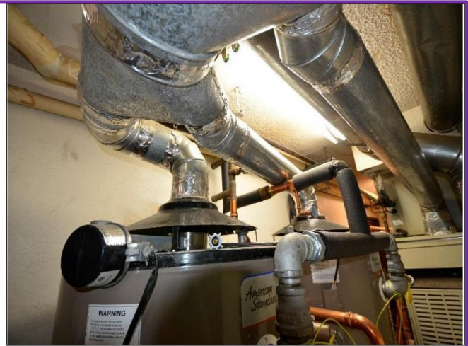
38. Exhaust flues have been properly installed with the proper slope angle to exit the exhaust gases.
