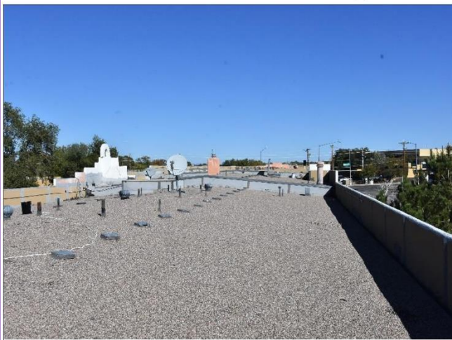
5. 1989 Portion of Roof is Hot/ Tar & Mop and is in better shape than the 1979 portion.
