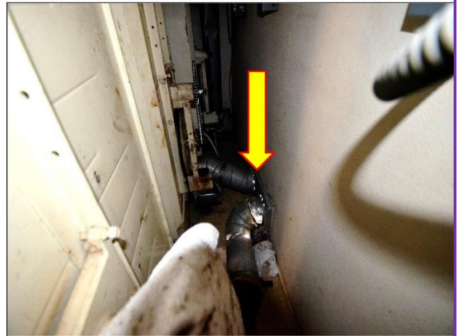
28. Ducting behind the Laundry Dryers for lint venting are badly damaged and will need to be replaced.
