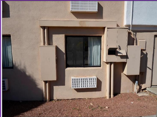
19. Electrical service wall on the East side will need to be verified by a licensed electrician.
