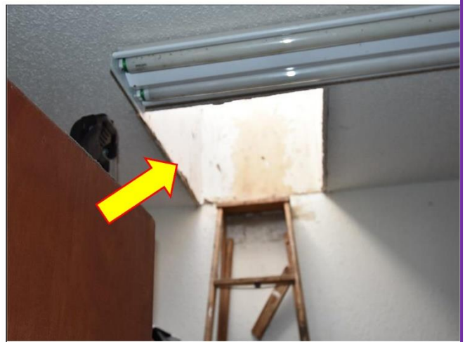
12. Hatch top the roof should have a better ladder for safety to inspect and maintained the roof.
