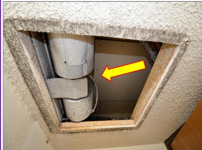
33. Inverter electrical heater for the Office in the Utility Closet's ceiling was NOT working at the time of the Inspections and will need service or replacing.
