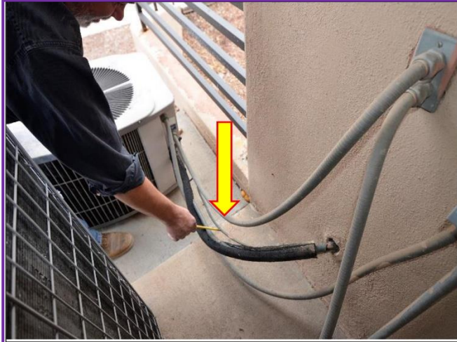
25. Condensers on the East side of the Building will need to be rewrapped with Armaflex insulation of the refrigerant lines.
