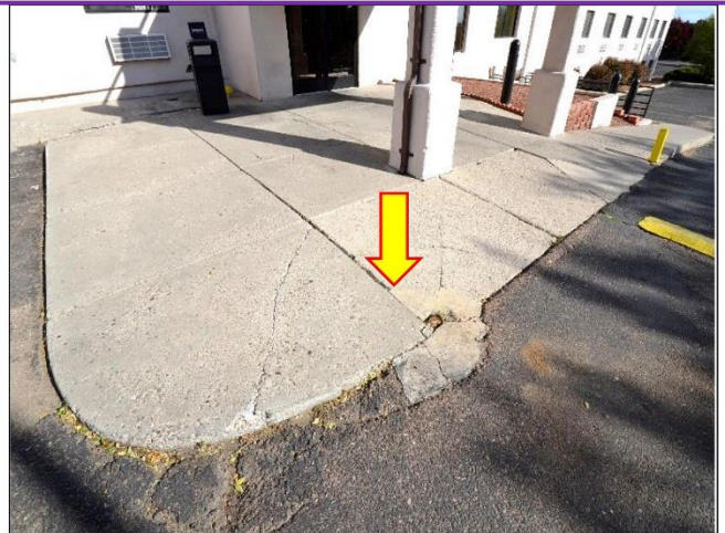
50. Concrete Flatwork is badly cracked in a few areas on the Entrance that can be tripping hazards and will need to be removed & replaced at expansion joints.
