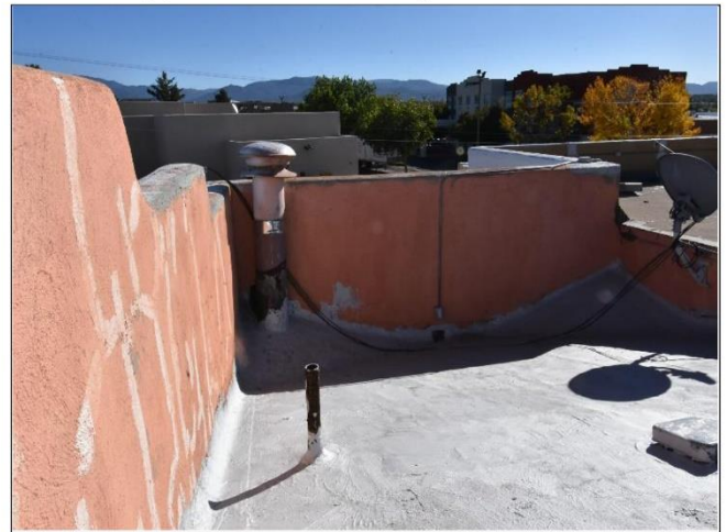
4. Upper roof section is a membrane roof that is sustainable for now and should be maintained at the same time as the rest of the roof levels.
