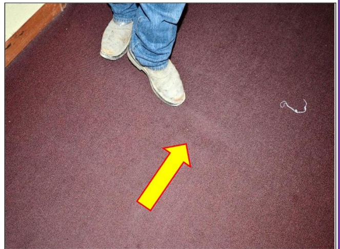
76. Hallways on the 1979 portion of the Building has many soft spots and seam separations under the carpeting that will need immediate attention.
