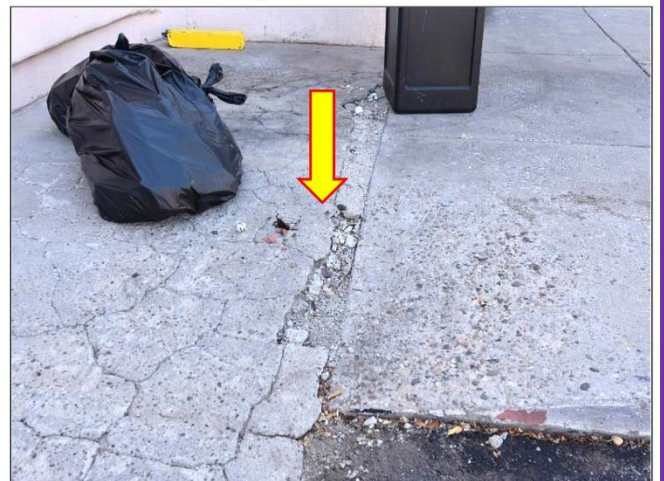
48. Example of broken Concrete flatwork that has deteriorated and will need to be removed & replaced.
