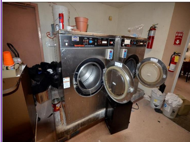
29. Two Laundry Machines found are working in good order.
