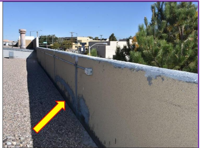
8. Parapets are Torch-down membrane and will need attention by a Professional Roofing Company.
