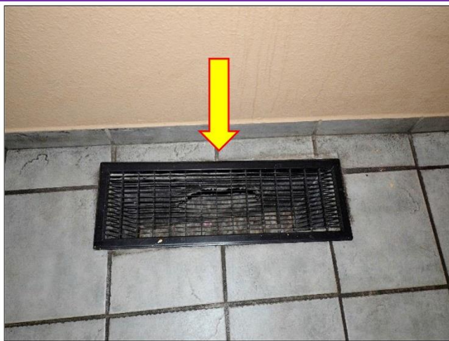
43. Downdraft vent found behind Lobby access area is for heating & cooling, but the register is loose and needs to be secured.
