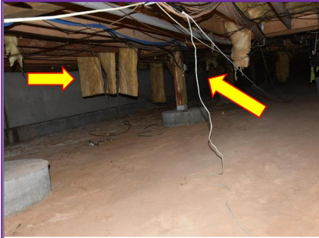
13. Under carriage of the building's Crawl Space will need attention to refasten the batt insulation and loose wires that have come loose.
