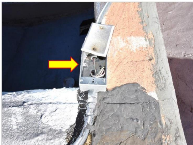
47. Example of Several electrical boxes that were missing cover plates and will need to be provided as per ICC & State UEC Codes.
