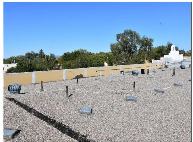
6. 1989 Portion of Roof is Hot/ Tar & Mop and is in better shape than the 1979 portion
