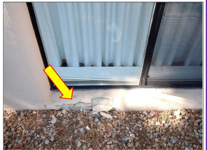
46. Windowsills at the Garden Level windows on the East side of the Building will need immediate attention for drainage and repairs to the stucco.
