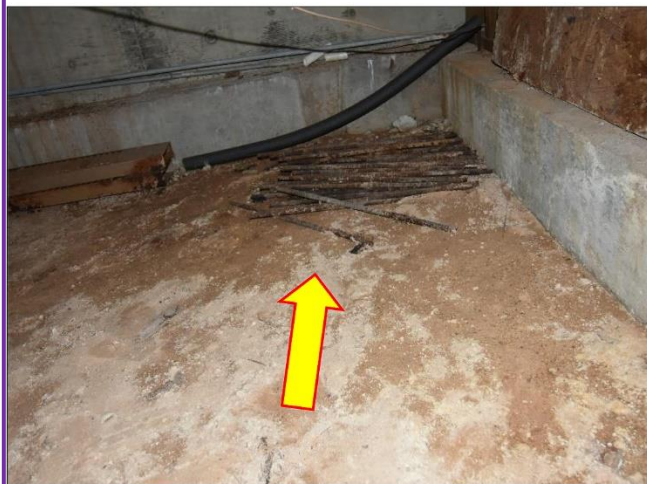
15. Moisture was found under the Crawl Space with water coming in from the exterior wall on the Northeast side that will need immediate remedies.
