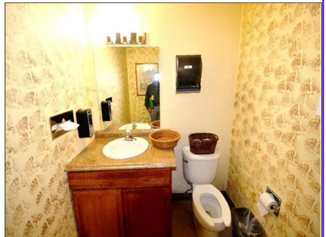
82. Public Bathroom is not ADA compliant without have grab bars, etc.
