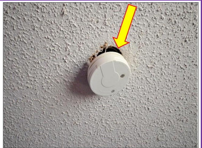
44. All Smoke Alarms throughout the Building and Guest Rooms will need to be Verified by a Licensed Electrician and Certified by the Fire Marshall.
