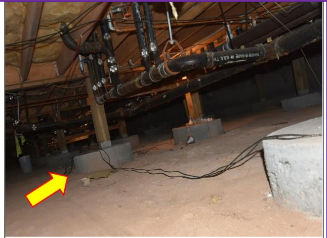
14. Crawl Space is showing a Platform type V-A construction with covered wood and supported by 4-rows of post-piers on circular concrete pads.
