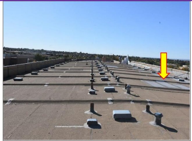
2. 1979 Portion of the Roof is Torch-down showing a lot of patching and will need professional reappointments in a timely manner.
