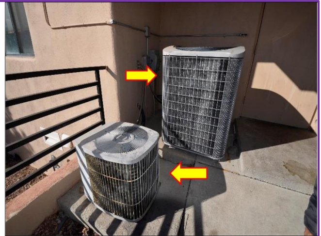
32. Two Carrier condensers found on the East side of the Building are for the Office, (smaller) and Lobby (larger) are for heating & cooling purposes.
