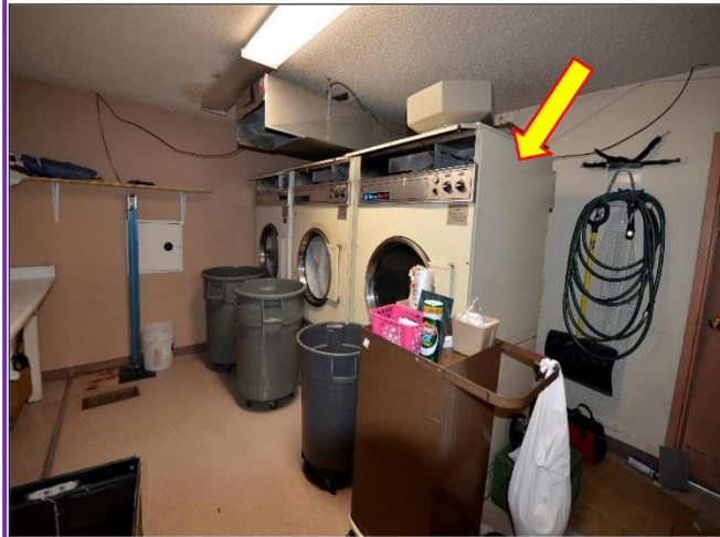
27. Three Laundry Dryers found, and one was NOT working at the time of the Inspection.
