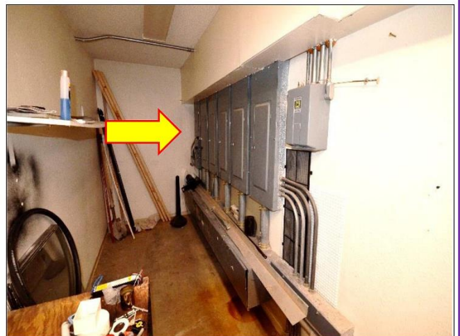
22. Five 200Amp panels found in the Service closet = 1000Amp Service to the 1989 portion of the Building. Better ventilation will be needed for this confined area.
