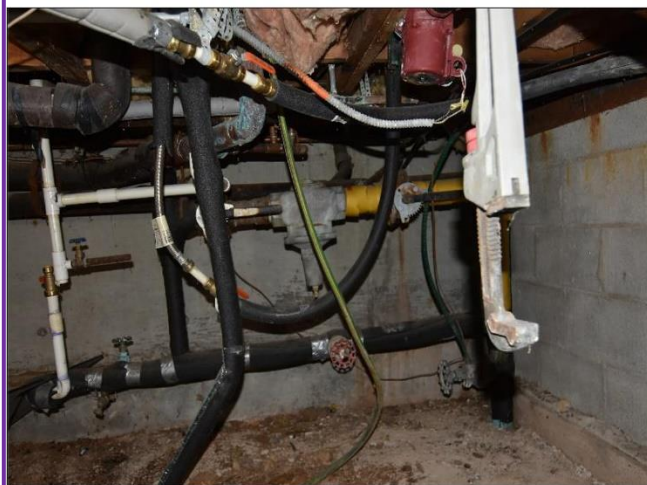
17. Plumbing pipes found under the Crawl Space seen to be reasonable with recent pipe wrap and without finding any other failures.
