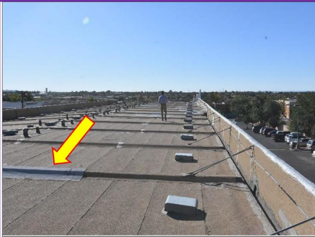
1. 1979 Portion of the Roof is Torch-down showing a lot of patching and will need professional reappointments in a timely manner.
