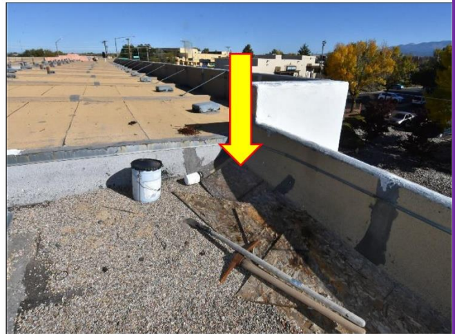
10. Debris and tools left out in the weather in bad and can cause deterioration of the membranes.
