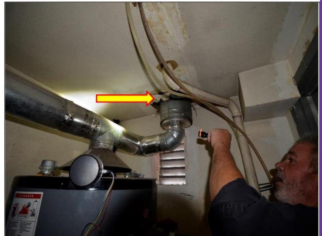
40. As per the Thomas' Report , the ceiling inside the Mechanical closet will need fireproofing and many other repairs.
