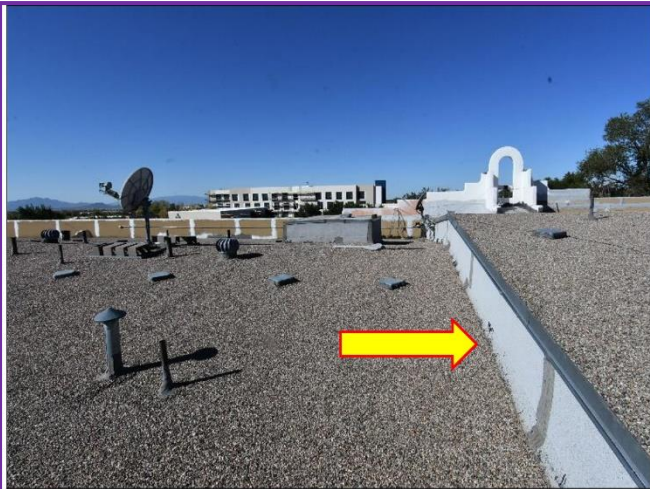
7. Parapets are Torch-down membrane and will need attention by a Professional Roofing Company.
