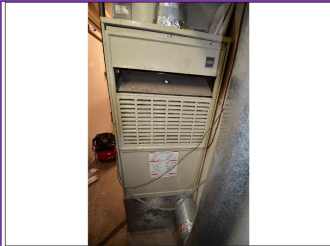
31. Carrier Furnace & AC Unit will need immediate Servicing by a Licensed trades' Professional. See Thomas' Report .
