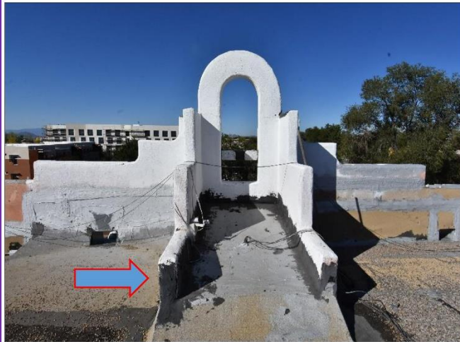
9. Faux Bell tower on the backside will need to be address with a Professional Roofing company because leaking may occur.
