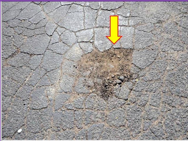
49. Asphalt driveway and parking lots have unraveled, showing alligator cracking and sinking potholes; will need a hot asphalt overlay and restripe.
