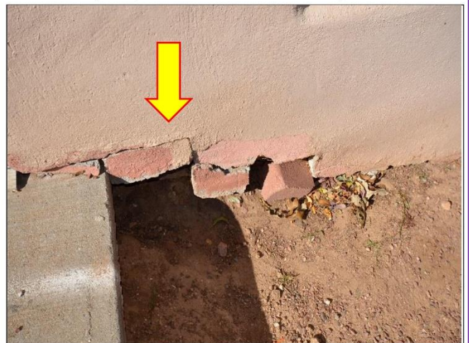
16. Water breach found on the Northeast side with loose bricks that are out of place with this type of construction should be removed with other remedies.
