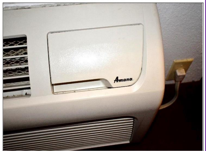
24. Typical Amana PTAK heating & cooling units are found in all Guest rooms and undergoing continuous maintenance and replacement as needed.
