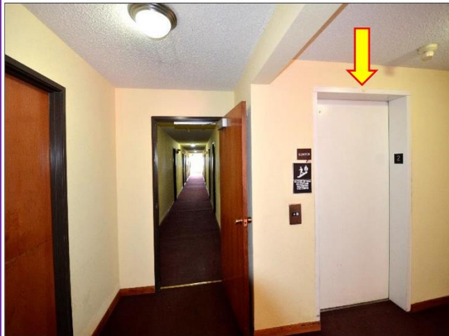
59. Otis Elevator, 30-feet 2 is for 3-floor levels was operating at the time of Inspection but will need to be Verified by Certified means.
