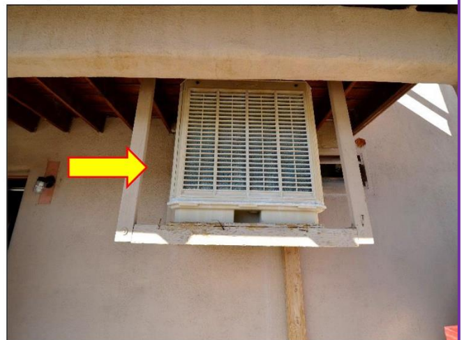
30. Swamp cooler found on the East side of the Building is for the Laundry Room only that will need annual servicing.
