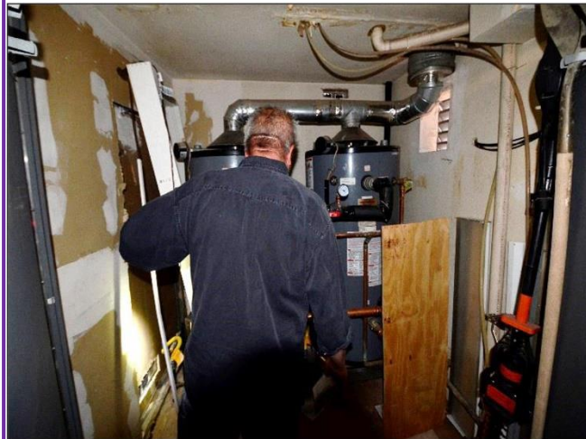
39. Mechanical closet having the two 100-gallon H 2 O heaters will need serious attention as reported by the Thomas' Report . Too much clutter in the room.
