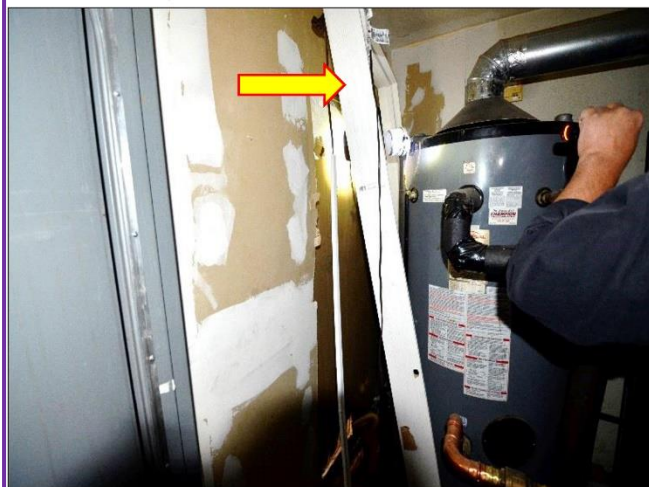
41. Mechanical closet having the two 100-gallon H 2 O heaters will need serious attention as reported by the Thomas' Report .
