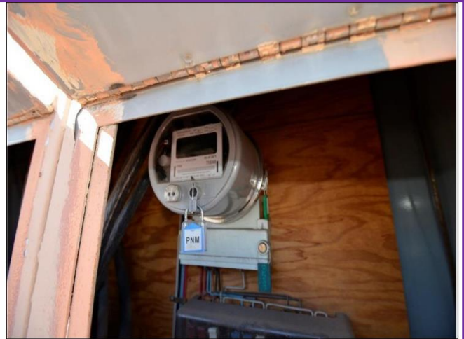
20. One PNM electrical Meter found on the East side of the Building has a cover door for readings.
