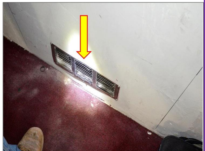
42. Outside Mechanical closet on the 1979 portion of the Building need immediate repairs as per the Thomas' Report . The vent is improper.
