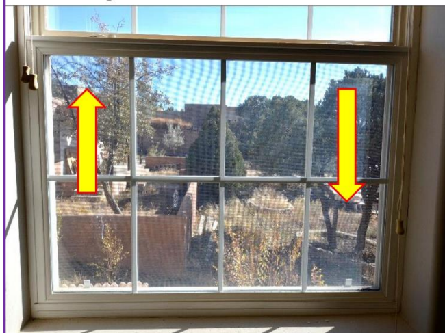
11. All of the vinyl Weather Shield Windows are difficult to operate smoothly and will need lubrication and adjustments by a Window Specialist.
