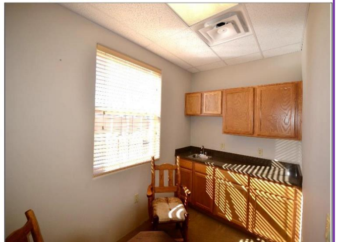
6. Breakroom with carpet floors, painted drywall, acoustical 9' drop ceiling and bar sink with cabinets is in Satisfactory Condition .
