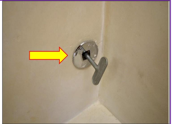
2. Gas valve to switchable Kiva Fireplace is badly stuck and won't open and needs attention.
