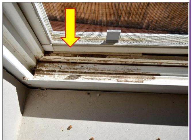
12. All of the vinyl Weather Shield Window tracks will need to be cleaned.
