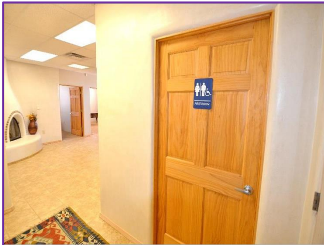
7. ADA Restroom with ceramic tile floors, painted drywall and acoustical 9' drop ceiling with toilet and wall hung sink is in Satisfactory Condition .
