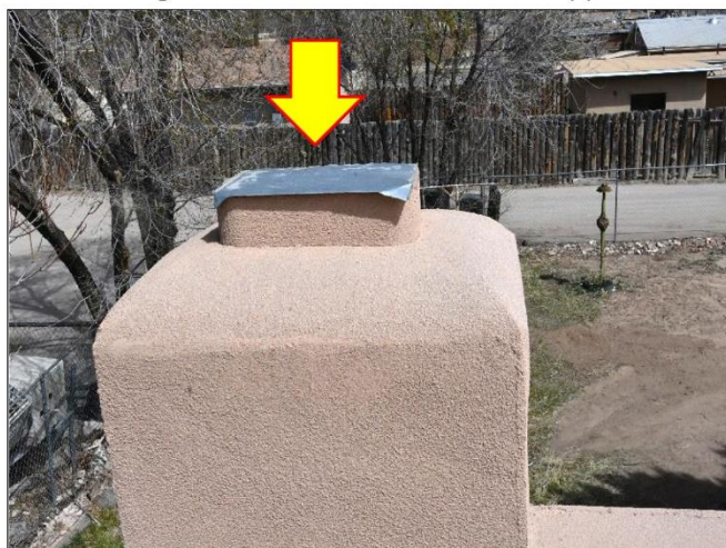
10. Kiva fireplace chimney is not set-up correctly will need a clay flue extension with a spark arrestor and rain cap as per City fire safety codes.
