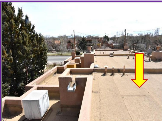
7. Torch-down roof has a longevity of 12 years and will need maintenance every 3-years for reappointments. Swamp Cooler is Winterized.
