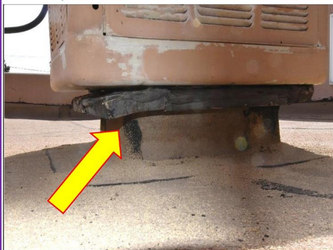
11. Chase under the Swamp Cooler looks like it might be leaking over the rooftop chase and this will need reevaluation by a roofing company.
