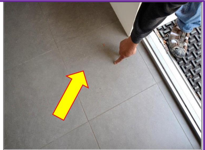
14. 4-cermeric tiles were found to be loose and sill need to be reset with adhesive.
