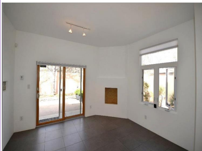
23. Living Room with Anderson sliding Patio doors and wood burning Kiva fireplace are in Satisfactory Condition .
