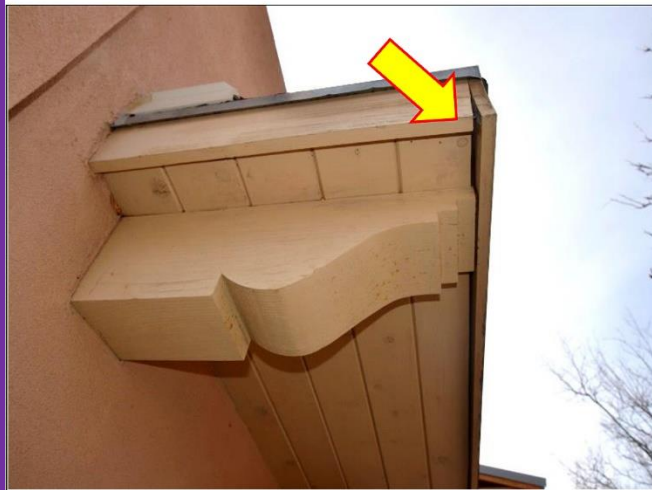
15. Fascia boards on both Patio door roof overhangs will need to be refastened and repaired.
