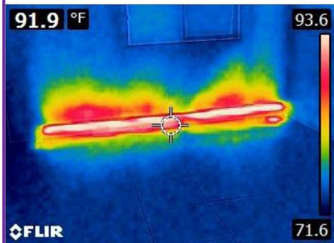
3. InfraRED Thermal Image on the Second Floor Level for hydronic baseboard heating without any flaws.
