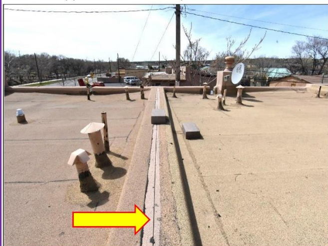
9. Firewall break between units will need to be reevaluated due to a continuous separation on top that will need to be covered.
