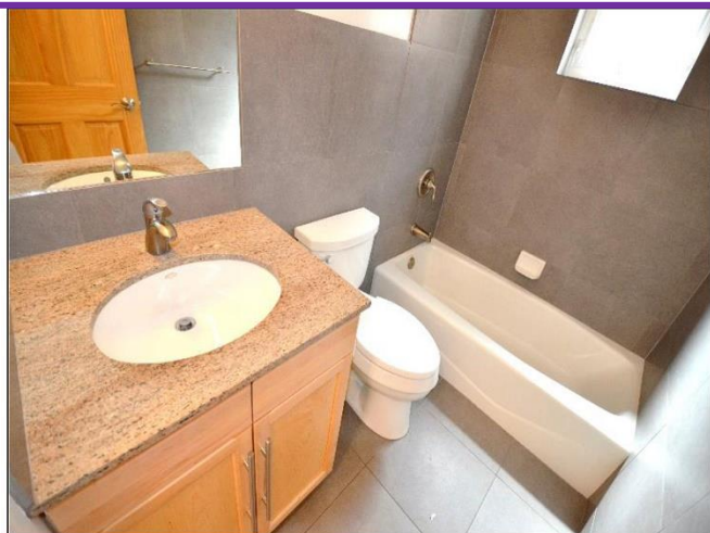
20. Lower level bathroom with Kohler fixtures/ vanity/ bathtub/ toilet are in Satisfactory Condition and are ASHI Verified.
