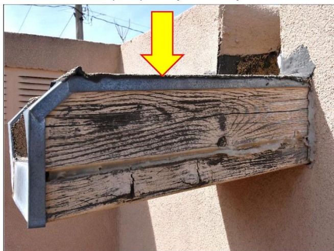
12. Typical wood canale will need to be refinished before taking possession of this Townhouse.
