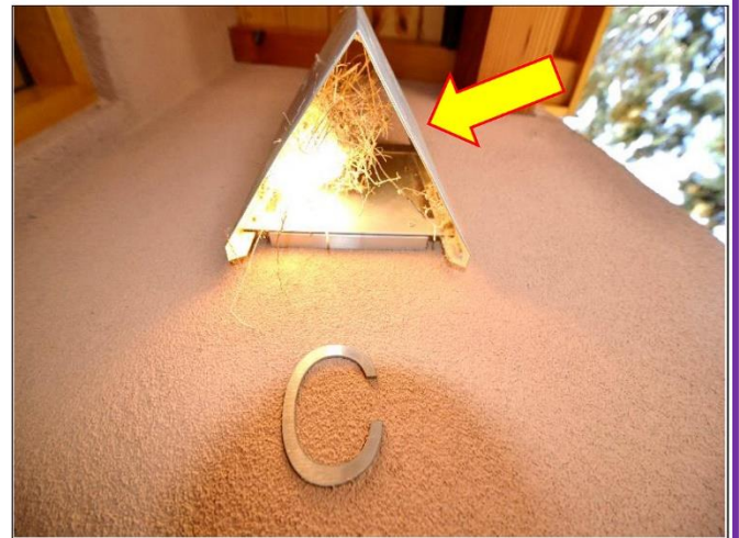
16. Birds' nesting found at the Front door light fixture will need to be removed.
