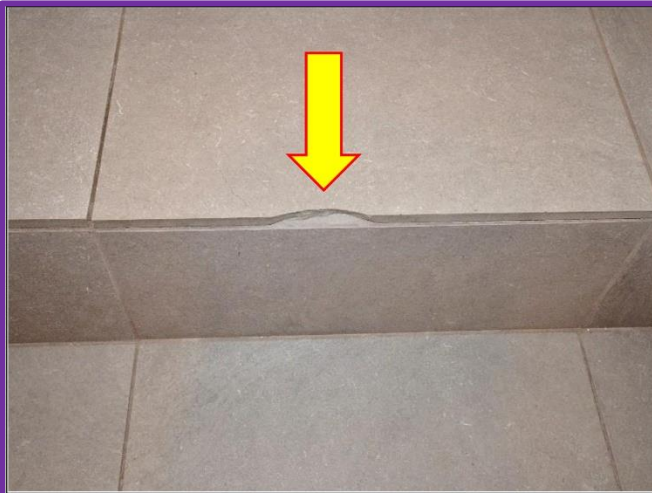
13. Chip found on tile tread to the Kitchen will need to be replaced.
