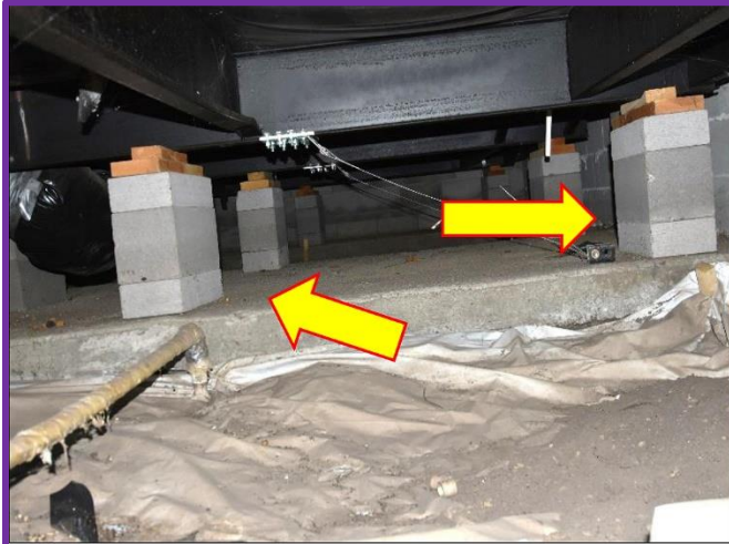
7. Crawl Spaces are properly built to support the Modular Homes but re-leveling might be necessary.
