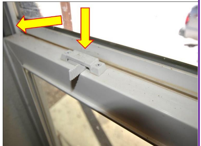
12. Some of the Window latches are not locking and will need further adjustments, track hardware replacements and lubrication.
