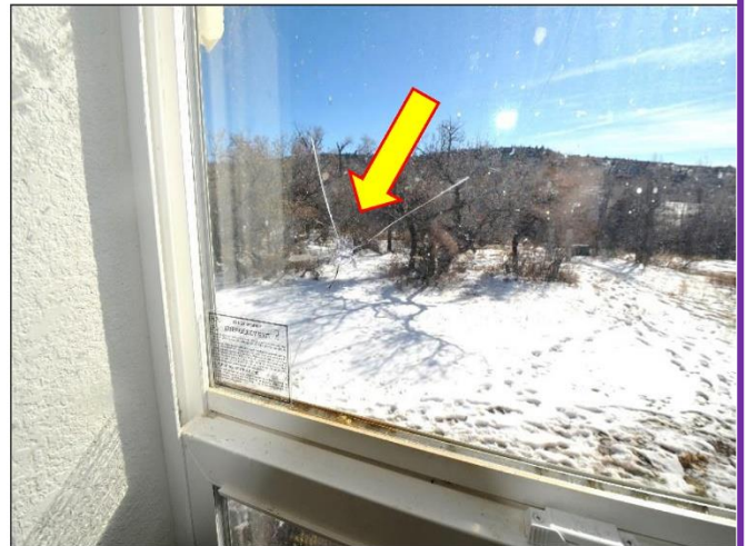
10. Broken window found on Master Suite Bedroom inside the First Modular Home that will need to be replaced.
