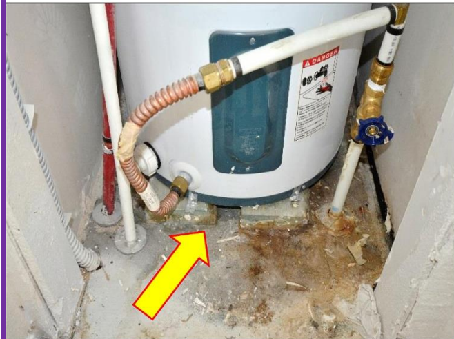
9. H 2 O heaters should have safety pans installed with drain pipes to an outside source.
