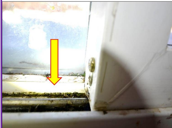
11. Sliding doors tracks on both Modular Homes will need to be cleaned and lubricated to operate properly.
