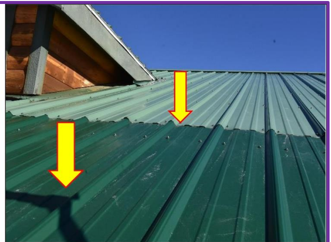
2. Propanel roof system is in Satisfactory Conditions except for this open gap with the panel replacement.
