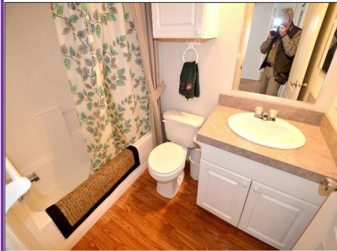
15. Both Bathrooms are in Satisfactory Conditions, except the First one need to have the heating register hook-up under the Crawl Space.
