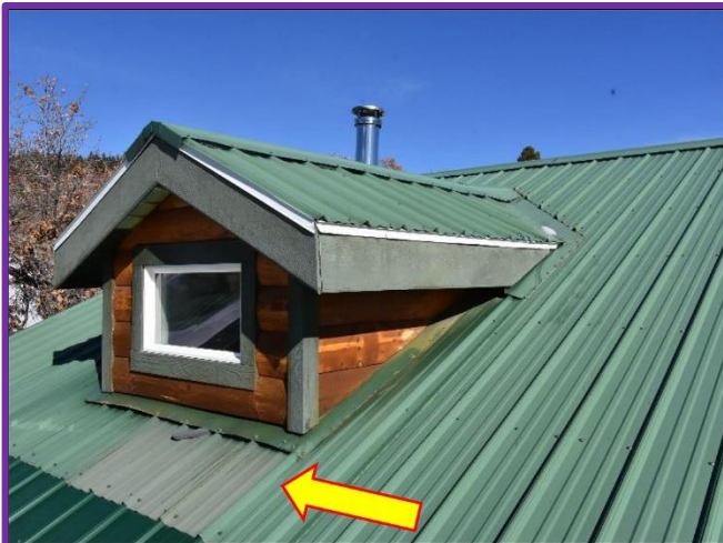
1. Propanel roof system is in Satisfactory Conditions but maintenance is needed every 5-years. Screws need to be checked to make sure they're secured.
