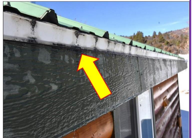
4. Fascia boards will need painted every few years and to be checked and/ or new angle trims should be installed to prevent wood rot.
