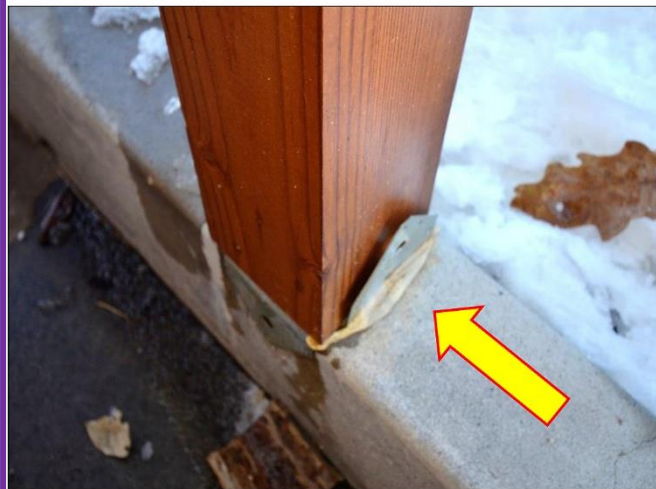
23. Example of Porch Post bases that should be nailed-off as per ICC and State UBC Codes. Glue is only a temporary solution.
