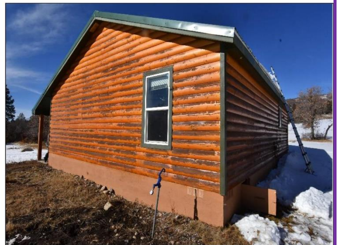
6. Split log siding will need to be re-stained to prevent deterioration.
