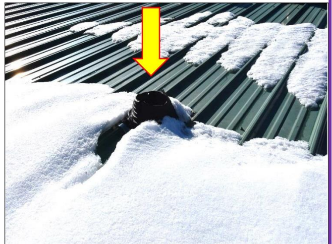
22. First Modular Home Bathroom roof jack for ceiling fan is open and needs the shaft pipe added to prevent leaking.
