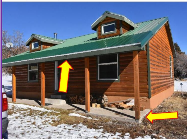
5. Porch post will need to be nailed at their bases as per ICC and State UBC Codes. Consider adding gutters and downspouts to control H 2 O run-off.
