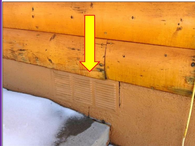
21. Foundation vent found on both Modular Homes space approximately 15-feet apart as per code.
