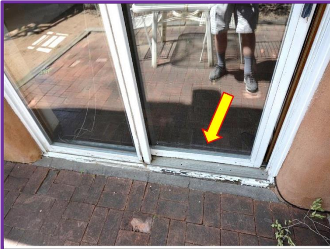
26. Casita sliding glass door units are falling apart and will need to be replaced.
