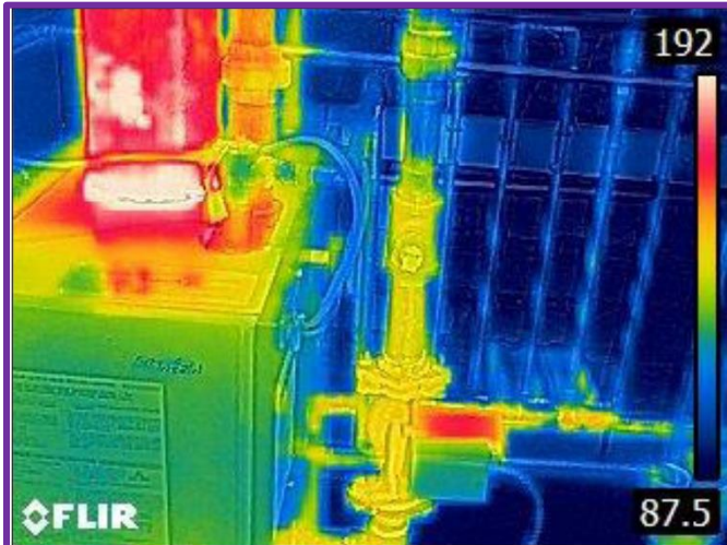
50. InfraRED Thermal Image showing mechanical SlantFin Boiler and 5-Zone valves are working in good order except for one Zone valve that isn't.
