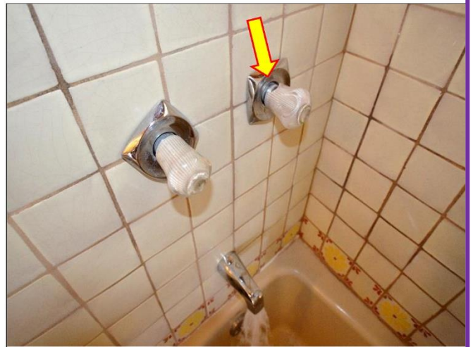
47. Casita shower knob is cracked and will need to be replaced.
