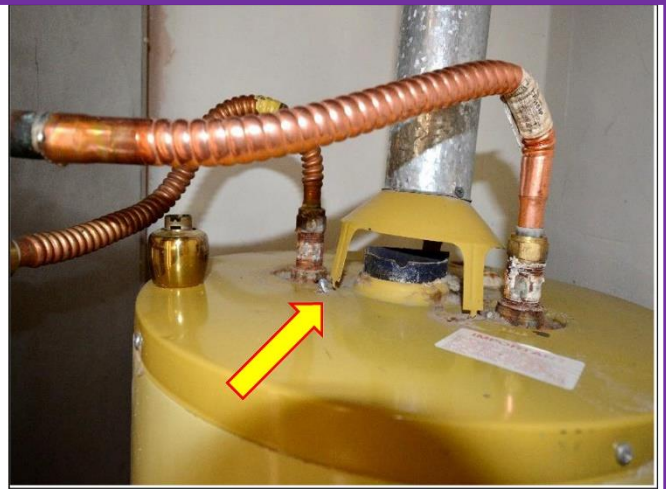
21. Casita H 2 O heater exhaust jacket is loose and needs to be secured to tank for CO safety.
