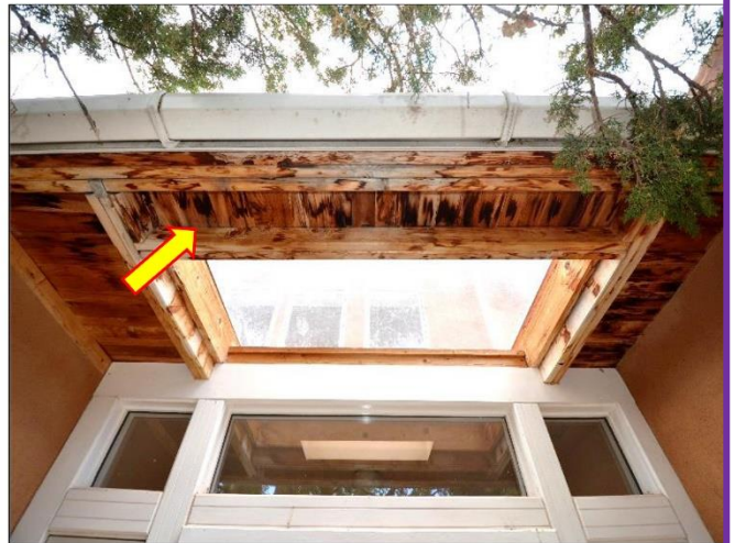
11. Water stains from prior leaking will need to be encapsulated with paint.
