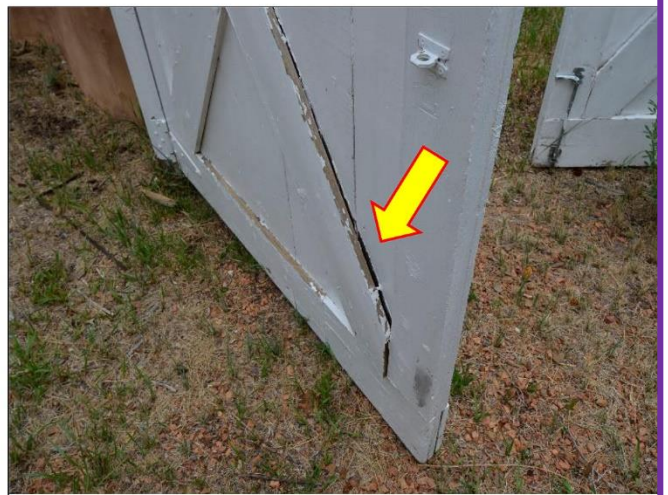
13. Gate Entry doors are rotting at the bottom and will need to have the wood components replaced and repainted.
