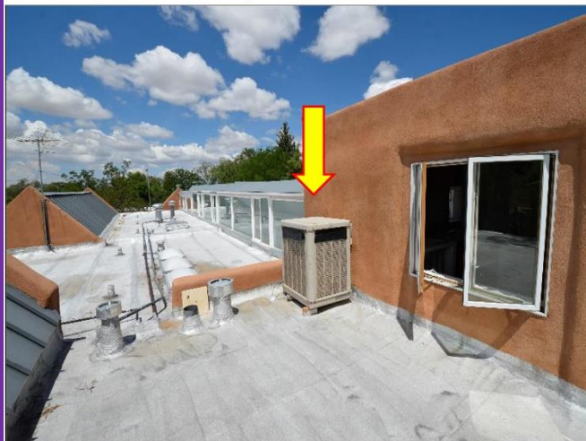
5. Swamp Cooler is not working at the time of Inspection but should be removed for a better cooling system such as with mini-splits.
