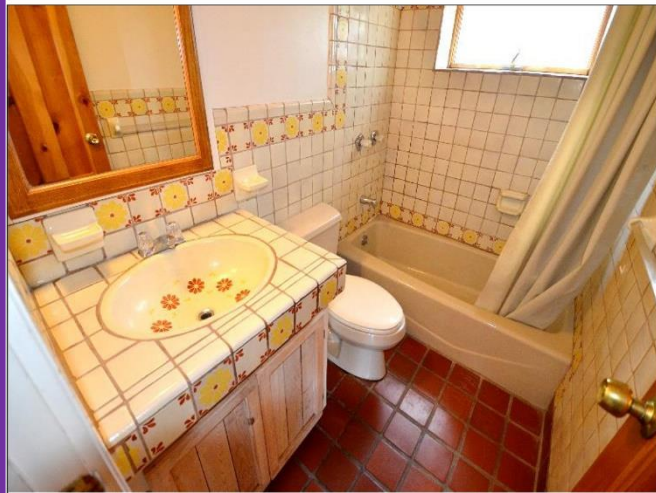
46. Casita Bathroom with Mexican tiles and ceramic tile floors are in Satisfactory Condition.
