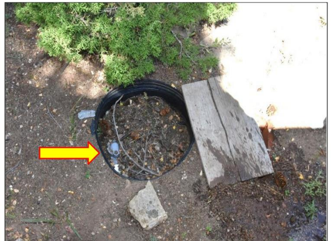
29. Access pit has a valve that is improperly covered by dirt and will need to be cleared.
