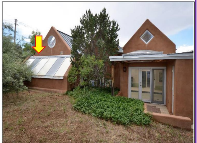
17. Plastic panels on the sloping walls are deteriorating and should be replaced.
