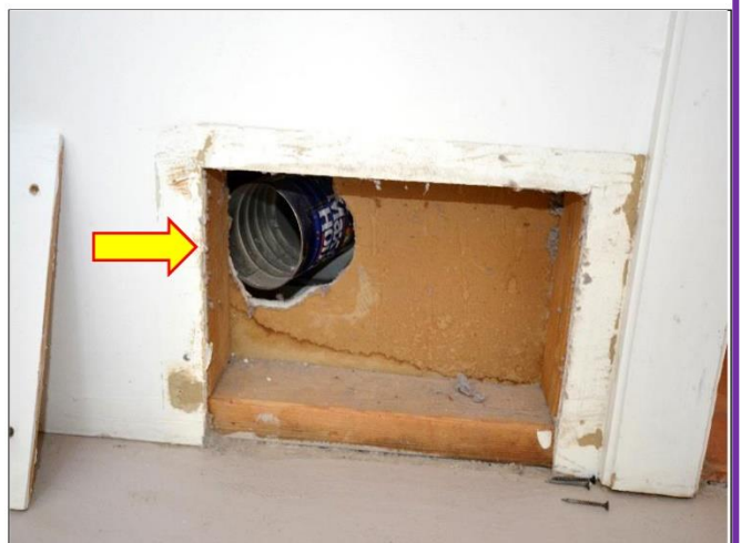
19. Coffee can was found behind the Laundry Dryer and is venting its lint into the wall cavity. It should be routed to the roof or to install a wall lint trap.
