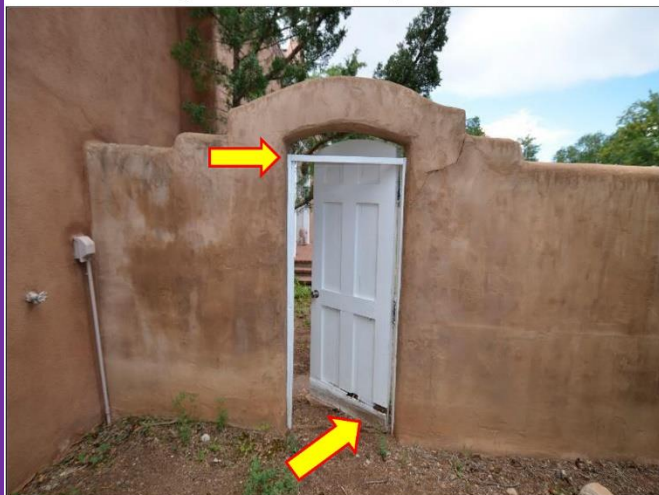
12. Gate door is rotting and will need to have the wood components replaced or replace the entire gate. Frame doesn't line up with the Gate.
