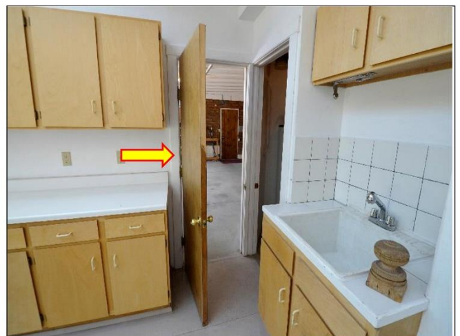
31. Rear door to Garage from the House is in Code violation and will need self-closing hinges as per ICC and State UBC Codes.
