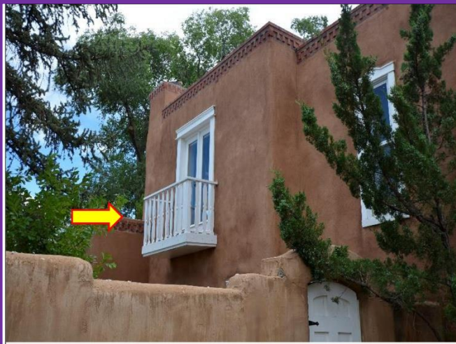
14. Balcony on the 2 nd floor Bedroom is in danger of pulling away from the wall and needs an architectural fix.
