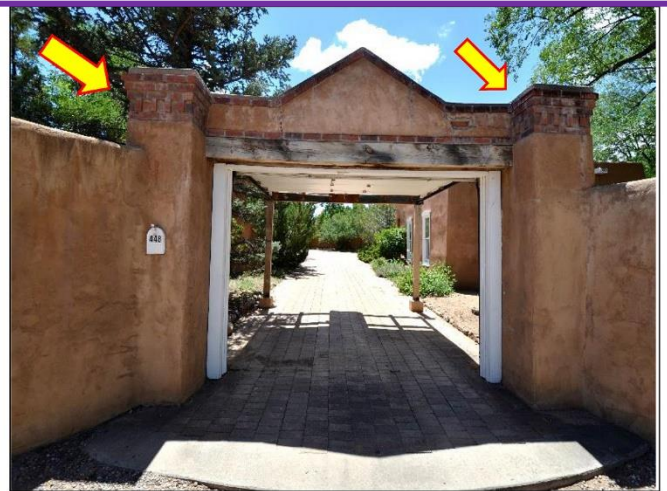
27. Territorial bricks above the wood arch beam are separating and will need to be repaired by a mason.
