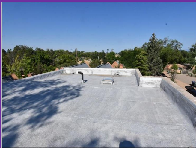
1. Torch-down roof membranes with a recent application of Aluminum fibers coverings on Main House & Casita are in Satisfactory Condition.
