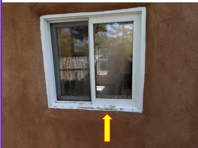
30. Typical window of many that need the trim repainted to prevent wreathing and rot.
