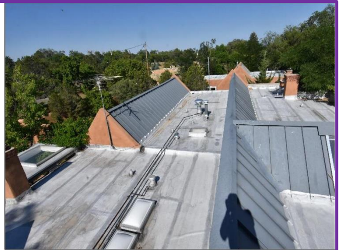
2. Torch-down roof membranes with a recent application of Aluminum fibers coverings on Main House & Casita are in Satisfactory Condition.
