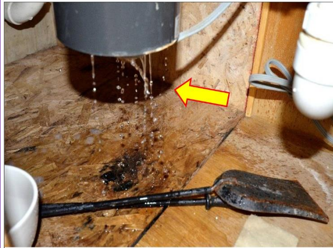
22. Casita waste disposal is badly leaking and will need to be replaced. Possible mold is present and will Remediation.
