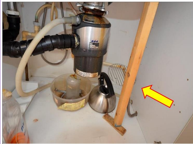
24. Prop stick found under Main House Kitchen sink is improperly holding up the stainless-steel sink and needs attention.
