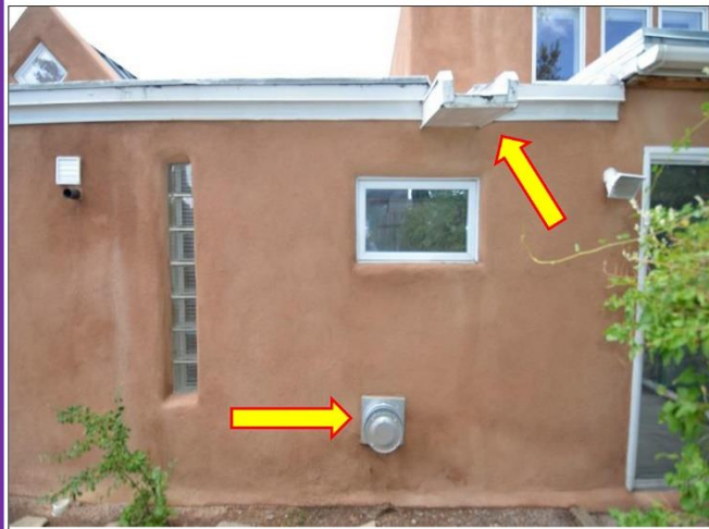
16. Bad arrangement having the exhaust vent below the window is a safety cod violation and it's not recommended to have a canale over a window.
