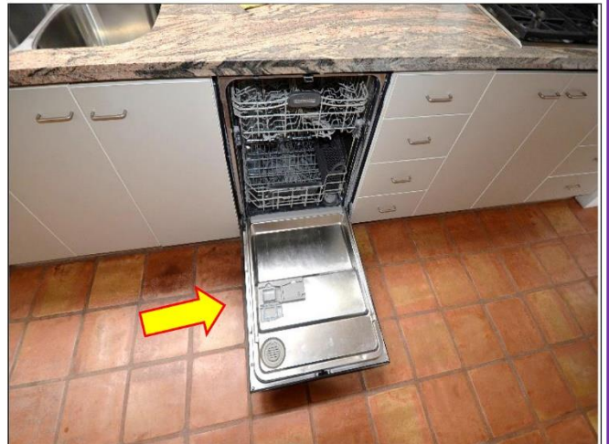
23. KitchenAid Dishwasher door on the Main House is broken and falling without having spring supports.
