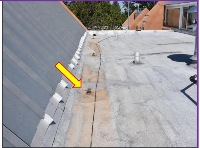
8. Drain openings on the roof above the Garage are too small and will clog because there are no leaf and debris grates
