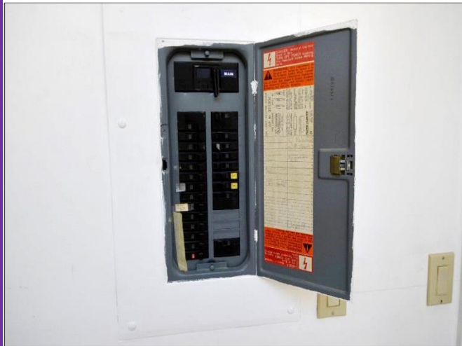
10. Main House 200Amp Electrical panel with labeled breakers and 3-subpanels were found throughout including Casita are all properly installed.
