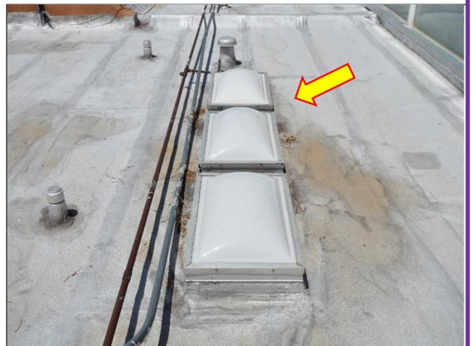
6. Row of Skylights can be replaced with one continuous hip type to better lighting.
