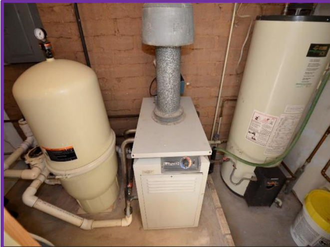
32. Swimming pool Mechanical equipment room with a separate H 2 O heater may be used to deliver hot water to the House and will need to be Verified.
