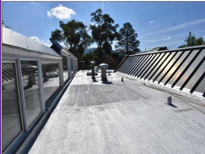
3. Clearstory windows and the high-pitched metal standing roofs are on the Main House & Casita are in Satisfactory Condition.
